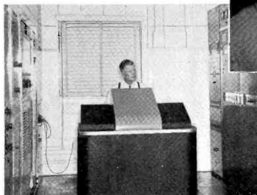
Control Room KDYL Transmitter
